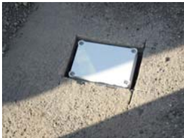
Fig. 4. Wireless sensor node embedded in road pavement
